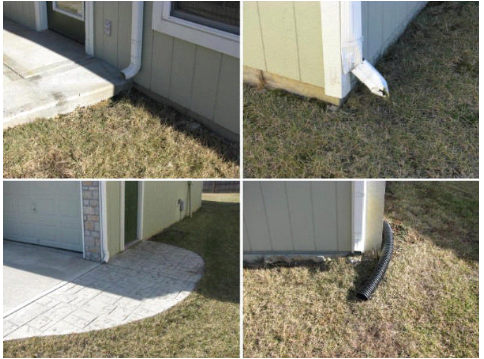
Downspout extensions are in need of repair / correction to direct water away from foundation at: North, South, West.
