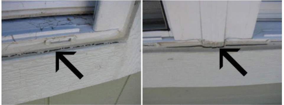
Caulking and sealing is necessary wherever weather can penetrate joints, cracks or other small openings. It is important to maintain caulking.
